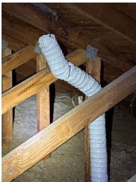
Exhaust vent terminates into attic
