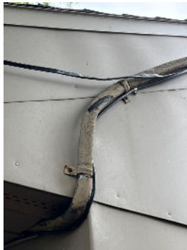
The service entrance wire insulation is deteriorated
