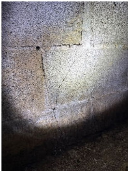
Settling crack observed on the east wall
