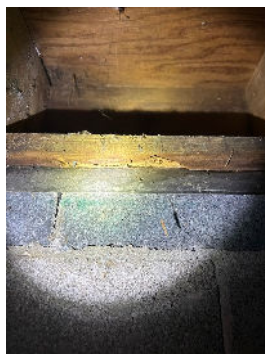
Heavily damaged sill plate from wood destroying organisms along the west wall. Approximately 8-10 ft worth
