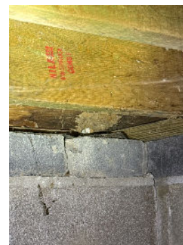
Non existent rim joists and damaged floor joist on the southwest corner
