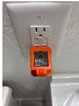
Outlet not properly wired
