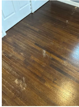
Worn/scratched flooring observed
