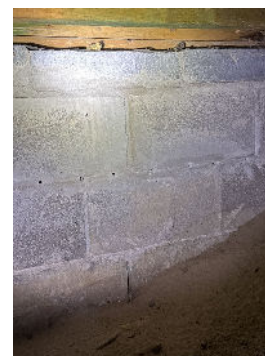
Additional evidence of wood destroying organism damage along the interior foundation
