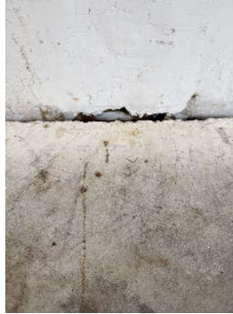
Damaged drywall along the south side of the garage
