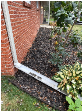
Negative grade on the northwest corner
