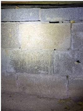
Shifted block on the south wall
