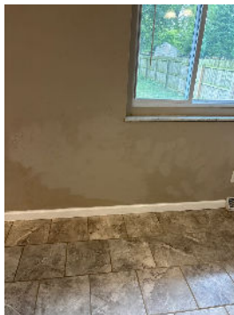
Poor repairs/paint job done on back wall
