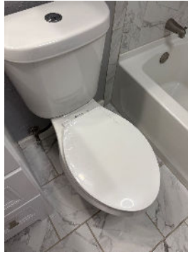
Toilet was slightly loose and will need secured
