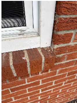
Multiple windows should be sealed again to the brick
