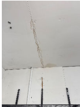
Moisture stained area observed
