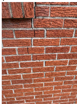
Mortar joint settling crack on the northeast corner
