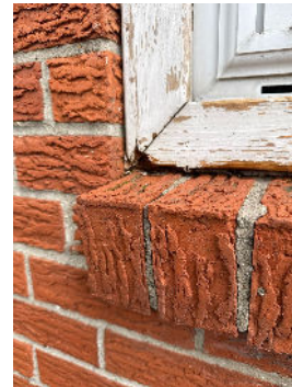
Rotten window trim on the northeast corner window
