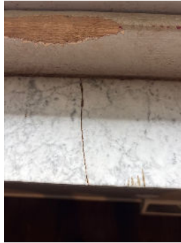
Window sill is cracked at front wall
