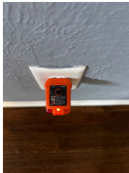
Open ground outlets in bedroom
