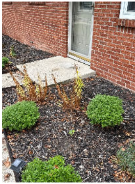
The front porch cap has sunk away from the home
