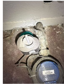
Missing shut off valve
