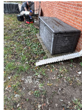
Negative grade on the northeast corner
