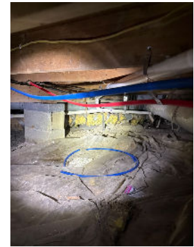
Loosely hanging supply lines observed
