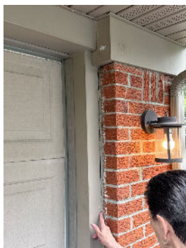
The trim around the garage door should be sealed again
