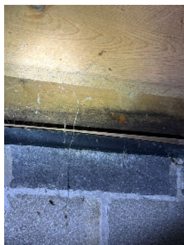
Mold like substance observed on the framing material on the northwest corner
