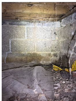
Significant shift in the foundation block on the north east corner
