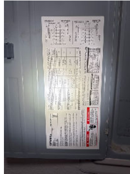
Electrical Panel Label
