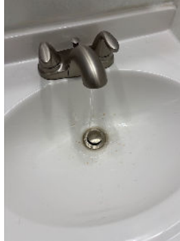
Low water pressure to sink when tested
