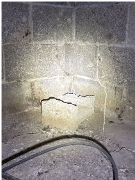
Pulled out/missing block on the south wall
