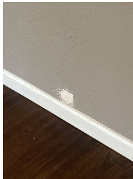
Poor repairs observed
