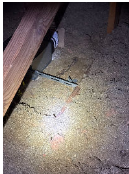
Missing insulation around exhaust vent
