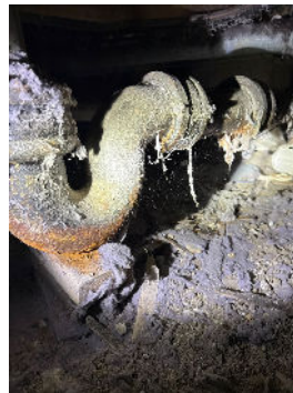
Several cast iron fittings are actively leaking
