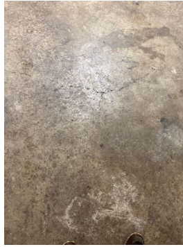
Common settling cracks observed
