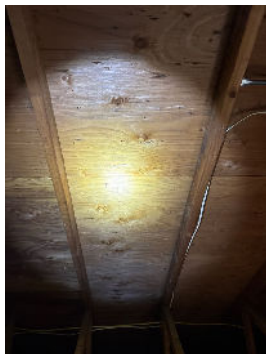
No H-clips installed on decking
