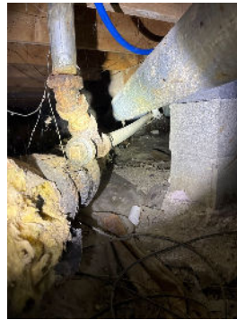
Improperly tapered drain line
