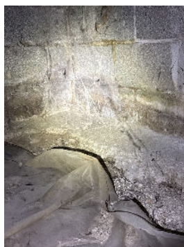
Efflorescence observed along the inside perimeter of the foundation
