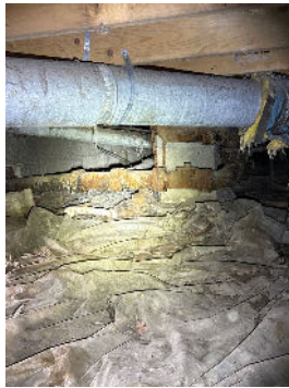
Improperly tapered main drain line
