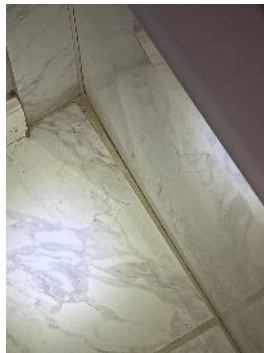
Tub isn't fully sealed to floor
