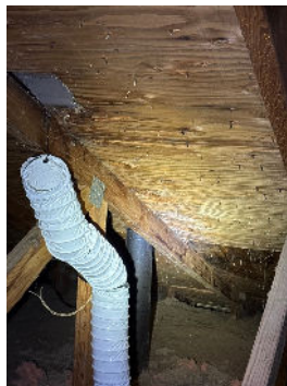
Evidence of previous moisture damage observed by exhaust vent. Slight sag observed in decking.
