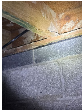
Cracked floor joist end on the east wall
