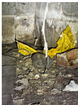
Active moisture intrusion on the northeast corner
