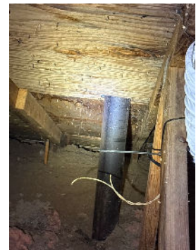
Additional evidence of previous moisture damage by soil stack
