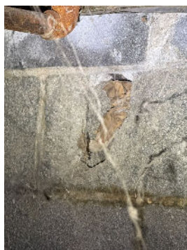
Damaged foundation block on the northwest corner
