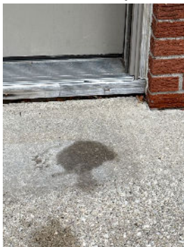
Small amount of chipped paint under the front entry door
