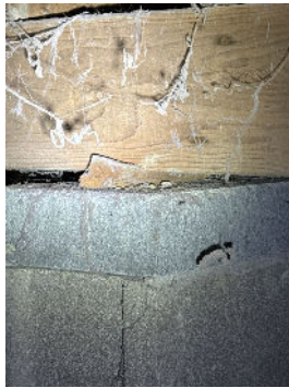
Multiple sections of beams have been shimmed with wood than have crushed
