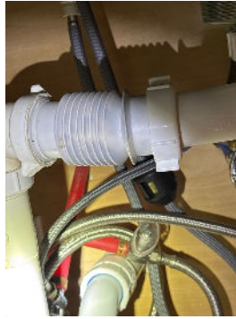
Flex drain observed for sink
