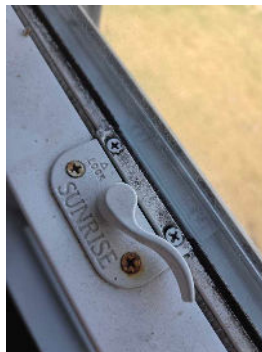
Mold like substance observed on window
