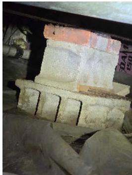
Improperly built column
