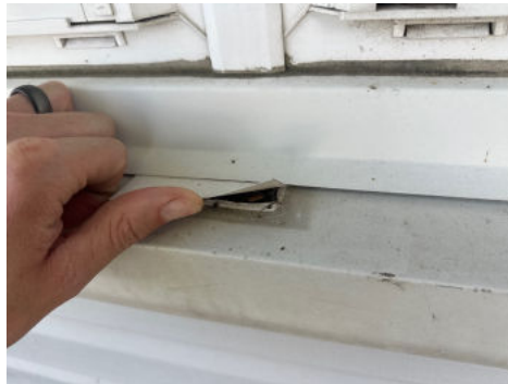
Improper trim repairs at windows
