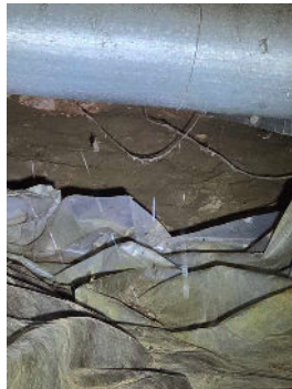
Missing proper vapor barrier in SE quadrant
