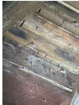
Additional evidence of mold like substance
