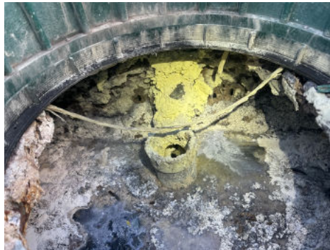
Significant deterioration at outlet end of tank
