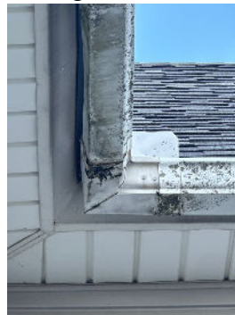
Loose and leaky gutters observed
