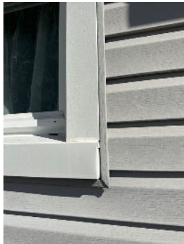
Windows need sealed to perimeter trim
