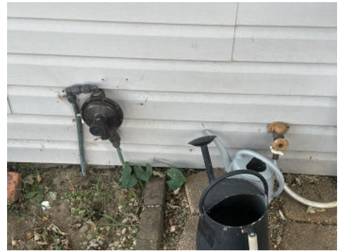
Siding penetrations and holes need sealed up at all times
