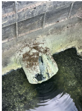
Cracked/damaged inlet pipe observed
