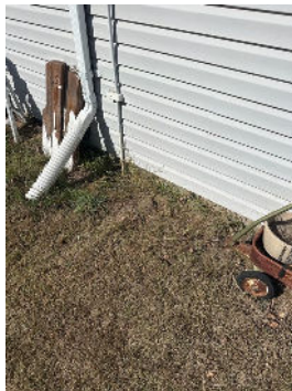
Low grading observed around home
