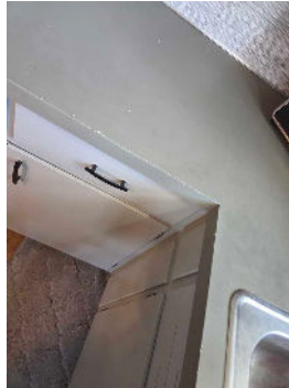
Worn countertop finish noted
