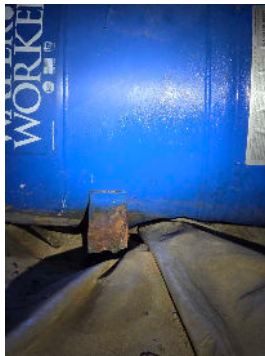
Corrosion observed on pressure tank.
