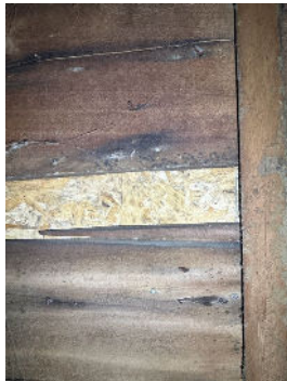
Mold like substance throughout framing
