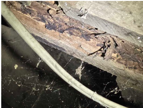
WDO damage observed
