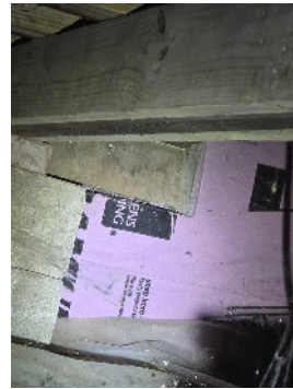
Vents have been blocked off
