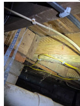
Missing joist hangers
