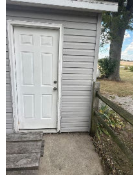
Loose wall observed at door.
