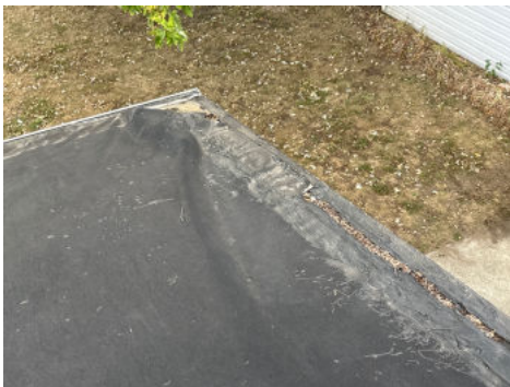
Rear rubber roof is damaged and needs replaced
