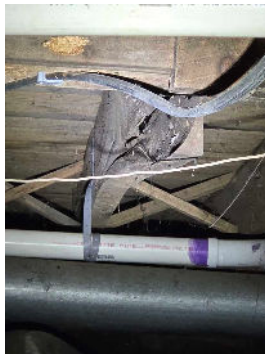
Cracked floor joist observed
