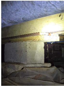
Wood shims observed under beam
