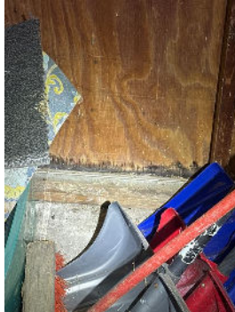
Active moisture observed at wall bottoms
