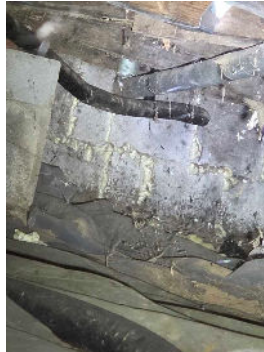
Missing insulation on east end
