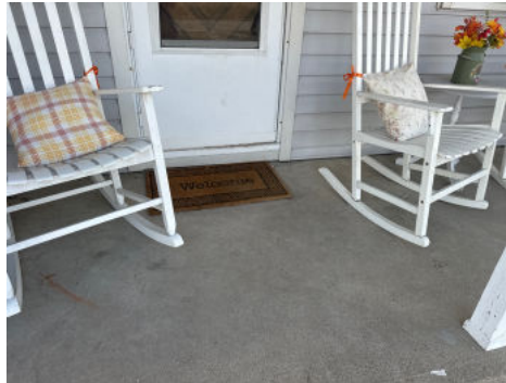
Front porch concrete needs sealed to home
