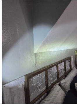
Poorly repaired section of wall observed
