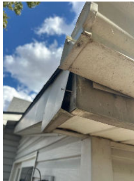
Loose trim observed at corners
