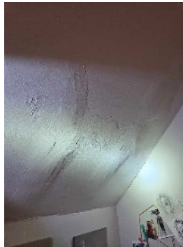
Poorly repaired section of ceiling observed
