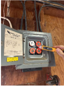
Live fuse panel in garage
