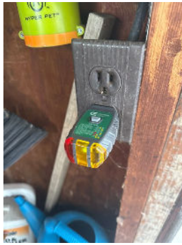
Open grounded outlets
