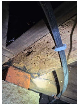
WDO damage observed on beam in center north end
