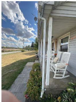
Gutters are loose from home and missing proper extensions
