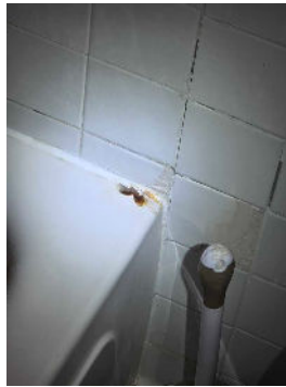
Deteriorated tub finish
