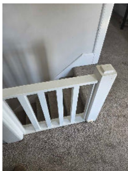
Guard rail does not meet vertical requirements
