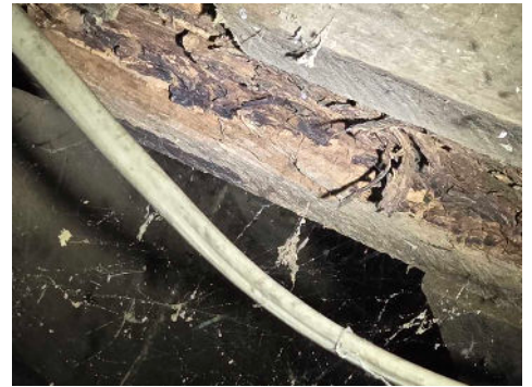
WDO damage observed
