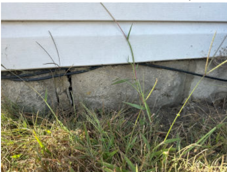
Mortar cracks observed at corners
