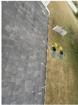
Southwest corner improper shingle repairs
