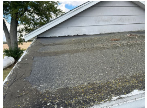
Improper tar repairs on backside of garage
