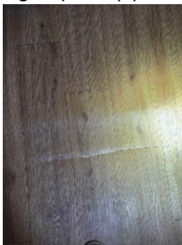
Damaged flooring material observed in doorway
