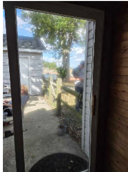
Patio door has lost its seal
