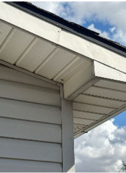
Transitions at corners need sealed up
