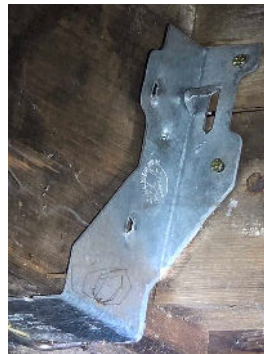
Hangers missing fasteners
