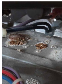
Corrosion observed inside furnace cabinet
