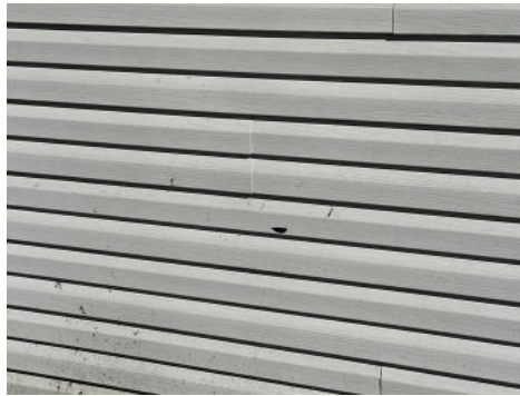
Damaged pieces of siding observed
