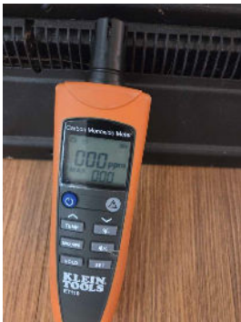
Carbon Monoxide Reading First Floor.
