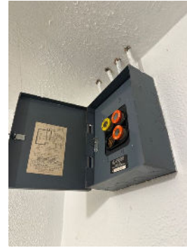
Additional live fuse panel in laundry room closet
