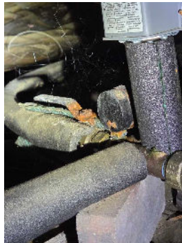
Corrosion observed on supply lines
