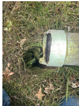
Cleanout to septic tank is broken/loose
