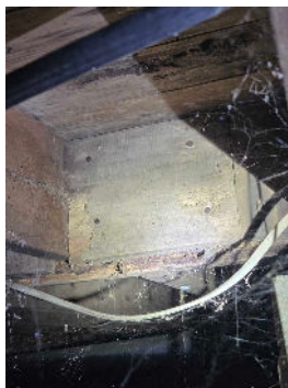
WDO damage observed to floor joists
