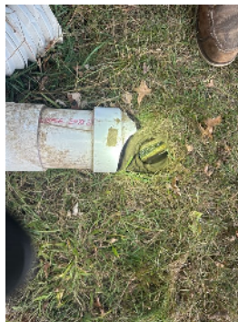
Broken cleanout observed near home leading to tank
