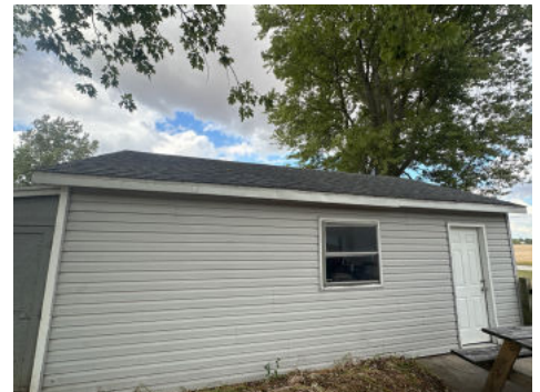
No gutters at garage observed
