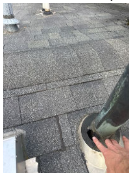
Multiple torn boots observed
