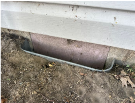
Vents have been blocked off
