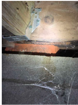
Rotten beam observed
