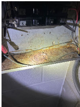
Corrosion observed in panel
