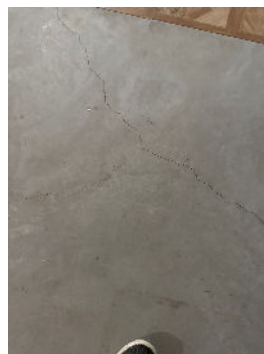
Common cracks noted
