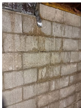
Stair stepping crack on the northeast corner
