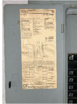
Electrical Panel Label
