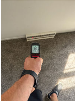
Warm Air Temperature Unit 1
