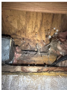
Termite damaged framing and subfloor on the north wall
