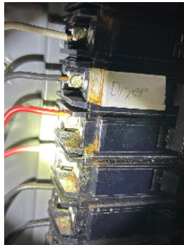
Corrosion observed on breakers
