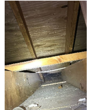
Evidence of previous moisture damage and rotten decking at the eaves in garage portion of attic
