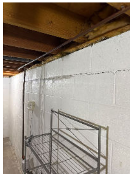
Small horizontal settling cracks long the east wall
