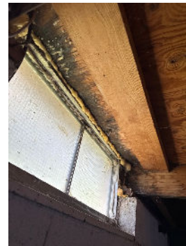
Small amount of rotten subfloor on the southeast corner
