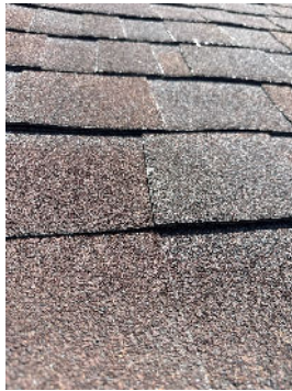
The fiberglass matting is exposed along the edges of the shingles indicating a roof near the end of its life
