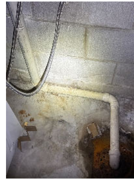
Efflorescence observed along the west wall
