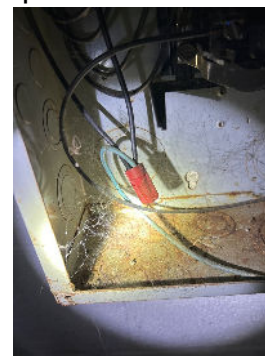
Triple tapped cable feed in bottom left side
