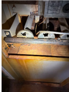
Heavy corrosion observed throughout the unit
