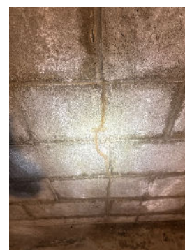
Termite tube observed on the north wall
