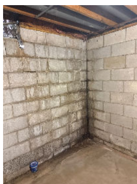
Active moisture intrusion along the entire north wall
