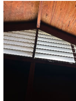
Gable end vent screen was missing on one side
