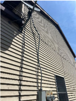
Service entrance wire isn't fully secured to the home
