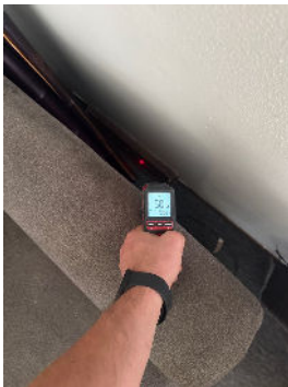
Cool Air Temperature Unit 2.
