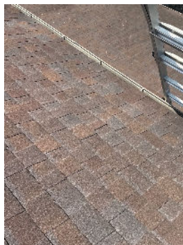
Several other soft spots observed along the eaves of the roof line
