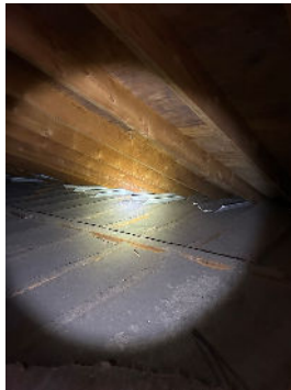
Majority of soffit baffles were not secured
