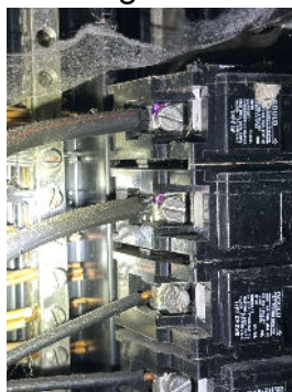
Missing anti corrosion paste
