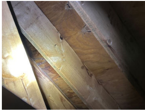
Evidence of previous moisture damage on decking in garage attic
