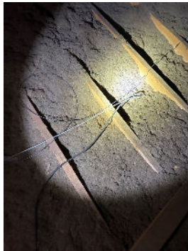
Multiple areas of minimal/missing insulation observed
