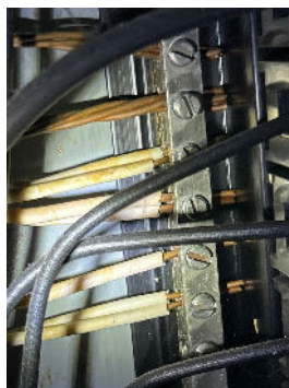
Multiple neutrals under same lug
