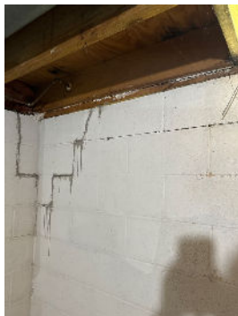
Stair stepping crack and small shift in the block on the southeast corner
