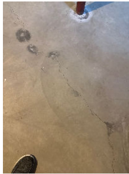
Common settling cracks noted
