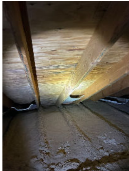
Evidence of previous moisture damage on decking on west side of attic
